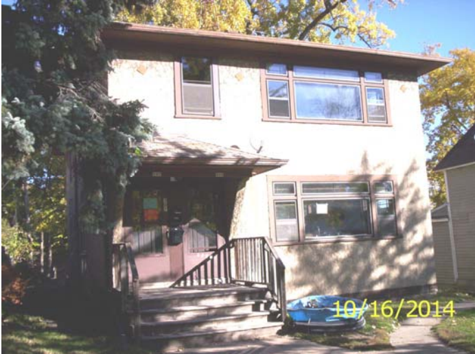
South and west sides, posting
