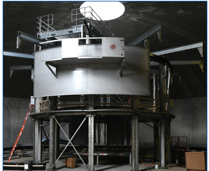
The inside of the clarifier on a tour of the new treatment plant held on May 24.
