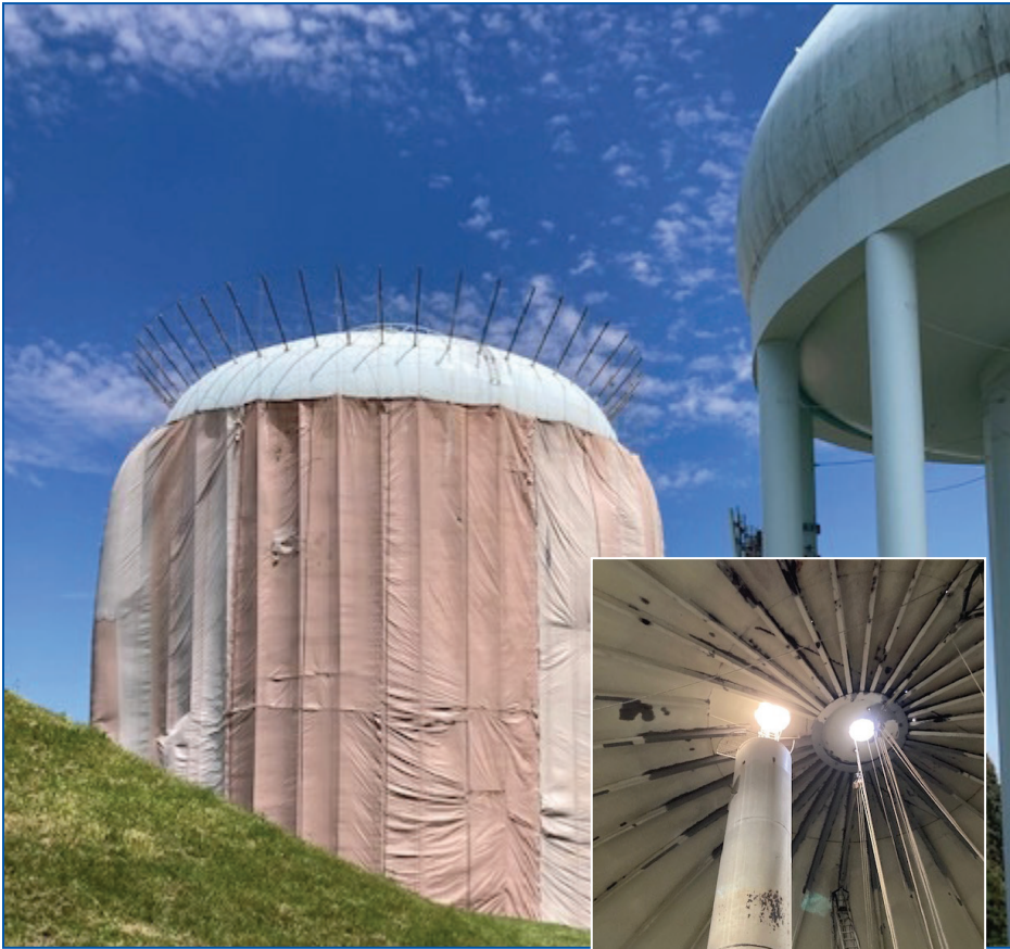
Highland water tank No. 2 gets sandblasted as part of the preparation for a new coat of paint gets underway on May 23. Photos by Todd Blomstrom.
