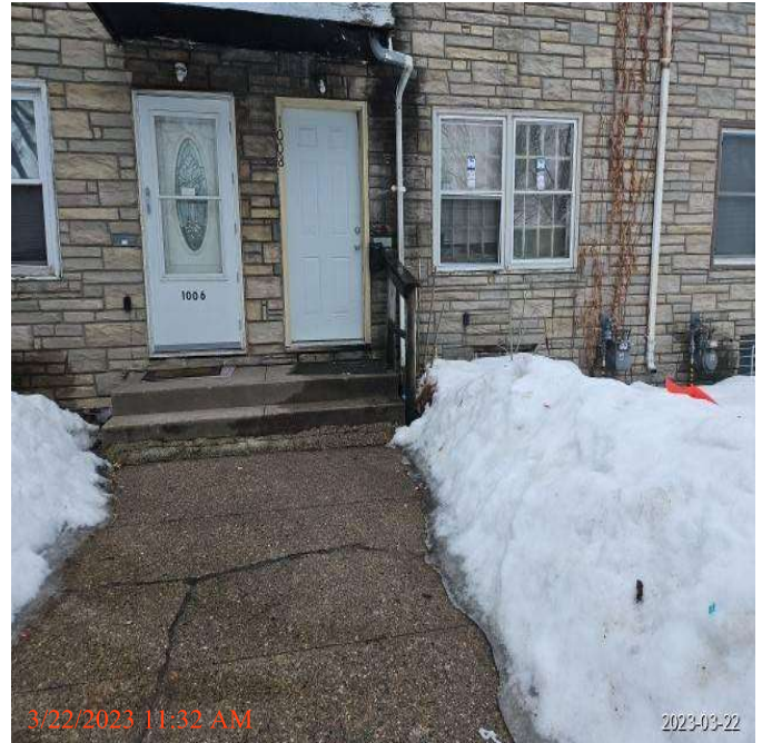
Address: 1008 CARROLL AVE SAINT PAUL MN 55104 Date Completed: 03/22/2023 Description: MISC other - exterior
