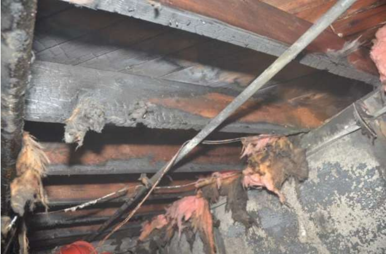
468 Thomas Ave.Fire Dwelling Photos 11-18-23
