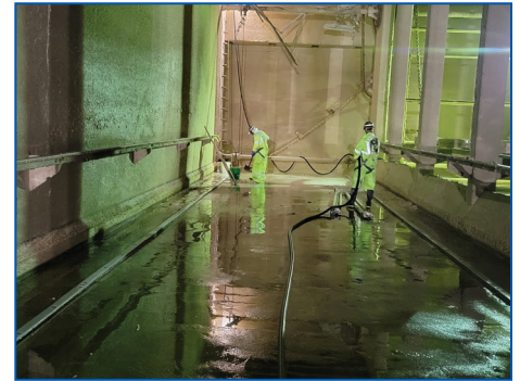
Workers clean out clarifier three after all of the chains have been removed from one section for repair.
