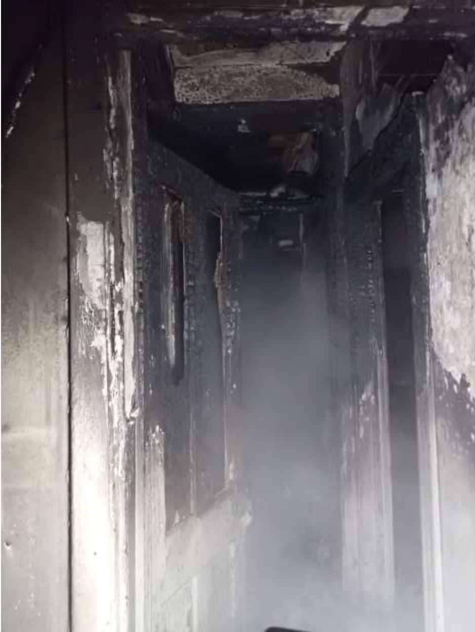
326 Charles Ave – Fire photos sent on 7/11/23
