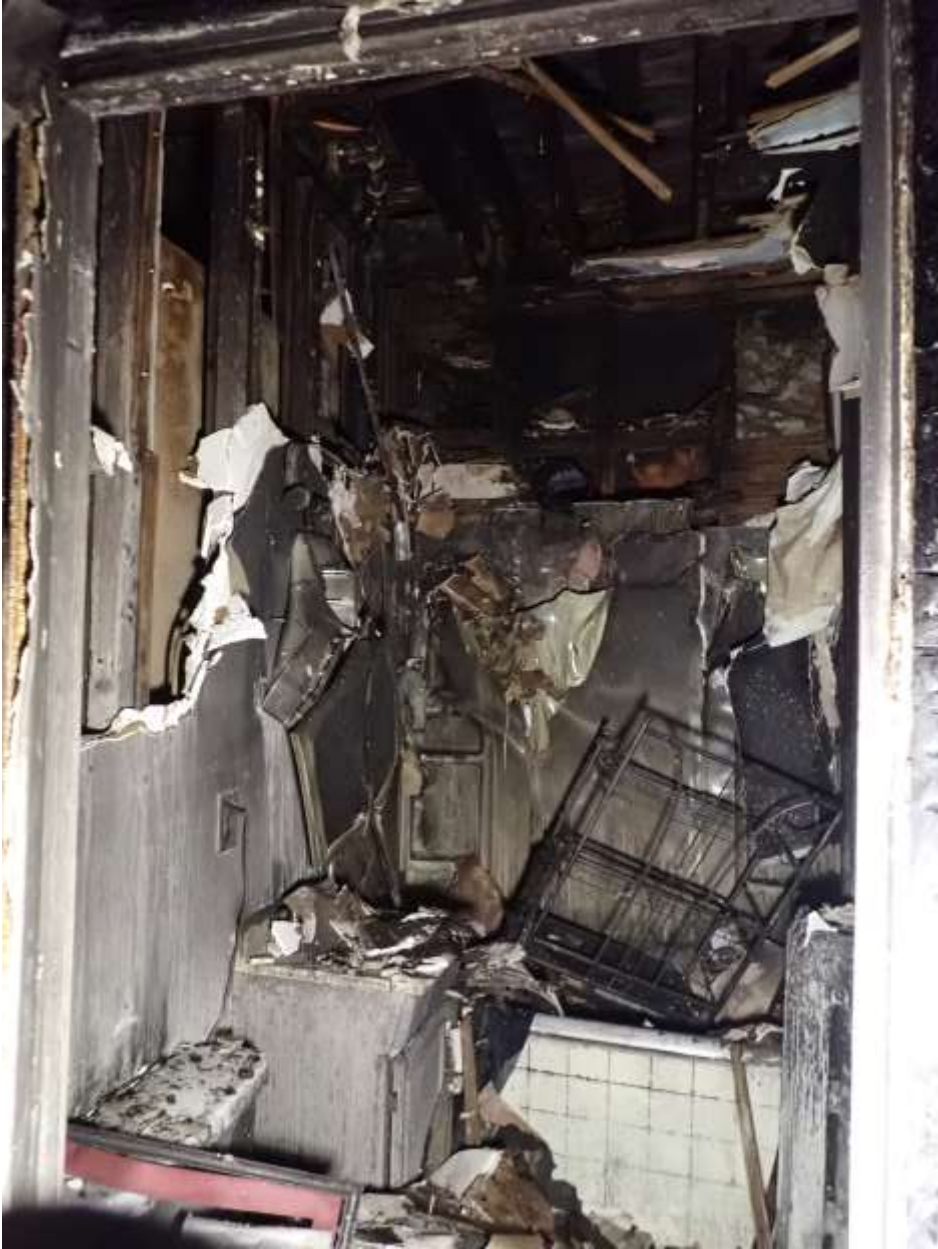
326 Charles Ave – Fire photos sent on 7/11/23
