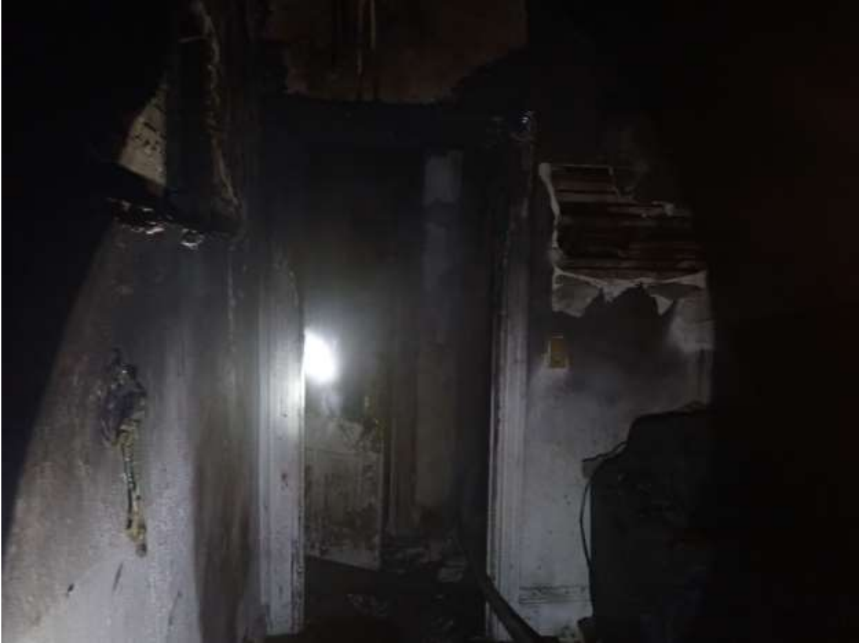
326 Charles Ave – Fire photos sent on 7/11/23
