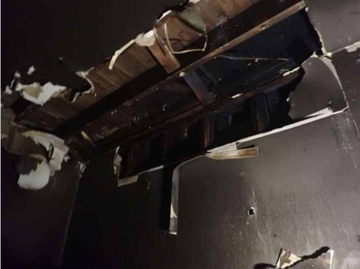
326 Charles Ave – Fire photos sent on 7/11/23
