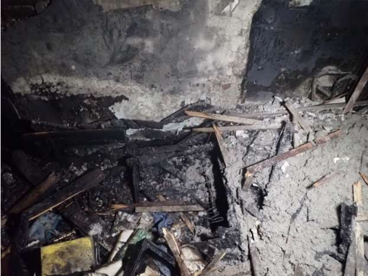
326 Charles Ave – Fire photos sent on 7/11/23
