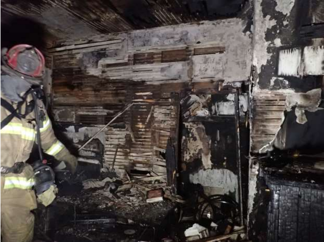
326 Charles Ave – Fire photos sent on 7/11/23
