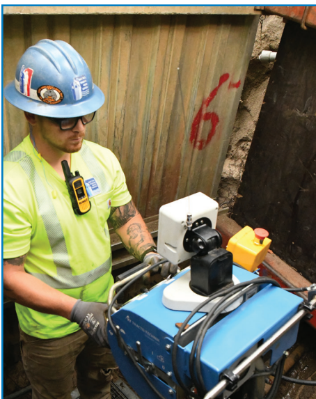
Jake O'Donnell runs the directional boring machine on a lead replacement on Randolph Ave. on July 11
