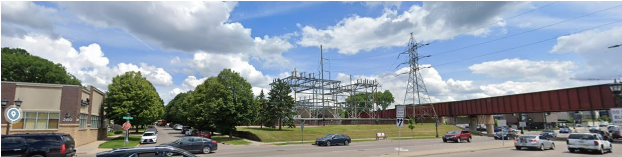
East of 271 Snelling Avenue North: electric transformer and railroad bridge over Snelling Avenue
