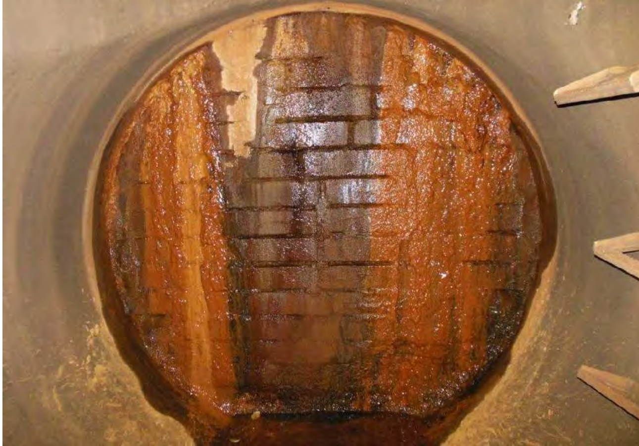
Iron Bacteria on Bulkhead
