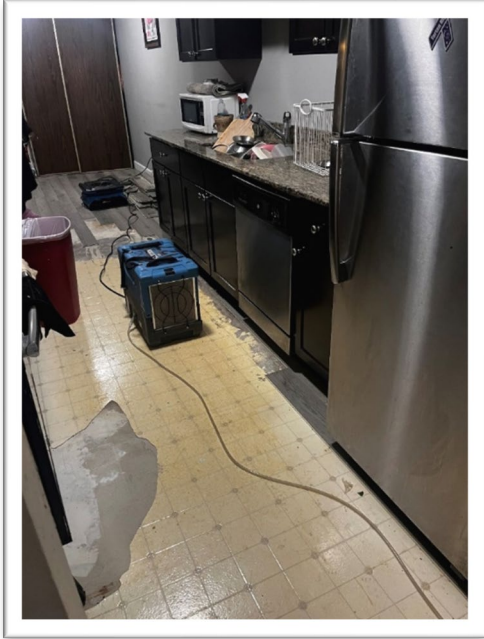
Above: Ripped faux tile vinyl flooring.
