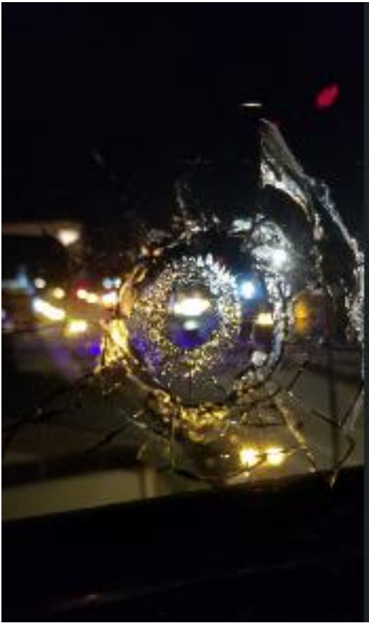
Bullet hole in kitchen window - 51 Grand Ave. 18 June 2022
