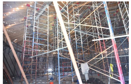
The scaffolding that supported the dome roofs in the clarifiers is coming out now that roofs have cured
