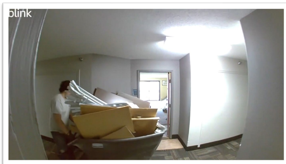
Carting uncovered demolition material in hallways after disturbance of suspect and presumed ACM.
