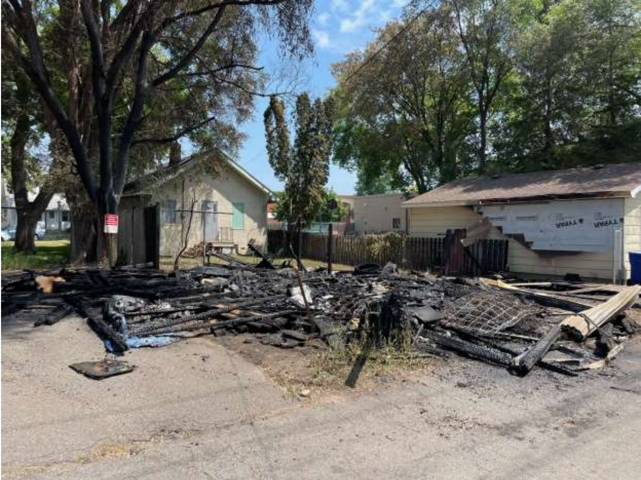
792 Rose Ave E. Garage fire 6/28/23
