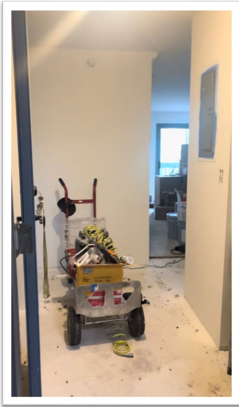
Screengrab from a video I took on May 22, 2023, showing renovation, including apparent floor and baseboard removal, being done in Unit 307.
