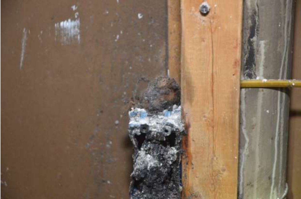
468 Thomas Ave.Fire Dwelling Photos 11-18-23
