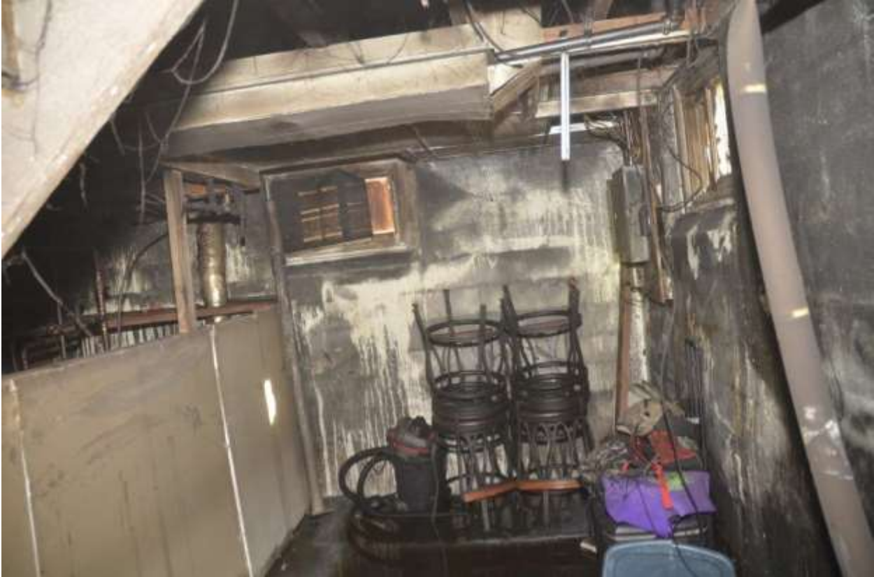
468 Thomas Ave.Fire Dwelling Photos 11-18-23
