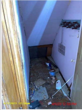
Photo: Bid Photos - Miscellaneous - 0085_2_After_App- Relocate interior debris personals.jpg Description: Bid Photos Description: ST0029866672
