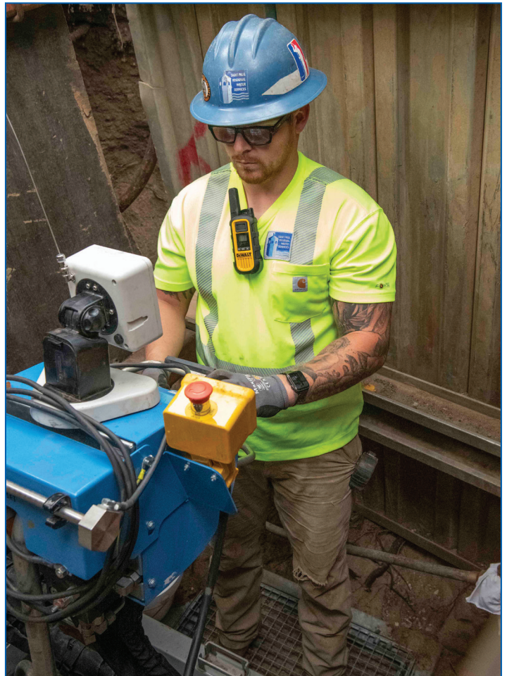
Jake O'Donnell, water utility worker, runs the horizontal directional boring machine on Lincoln Ave. Sept. 21. Some lead replacement crews started using the new machinery on Sept. 20. The machine operator can track and guide the drilling head through the ground, resulting in more accuracy than a pneumatic bullet. It can be used to drill directly into a home, after which the copper piping is attached and pulled back to connect to the water main or copper service line.
