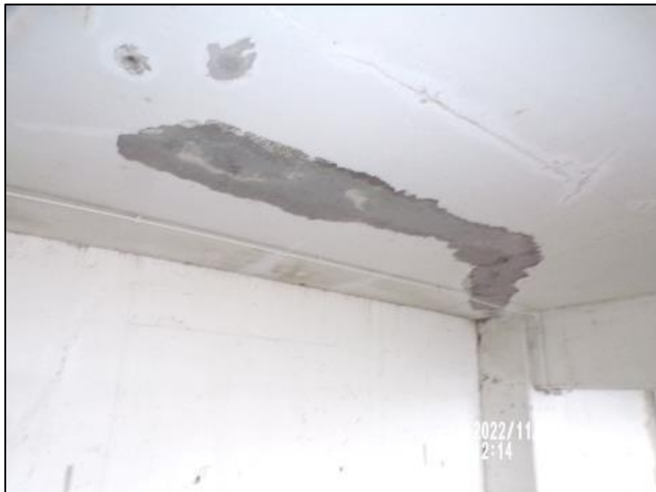
Bottom of slab cracks intersecting beam-column connection at foundation wall.
