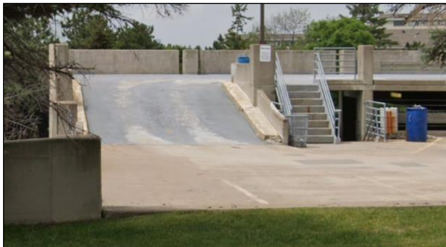
SK-3: Google Image of South Vehicle Ramp Between Levels 3 and up to 3 ½. Stair A next to ramp
