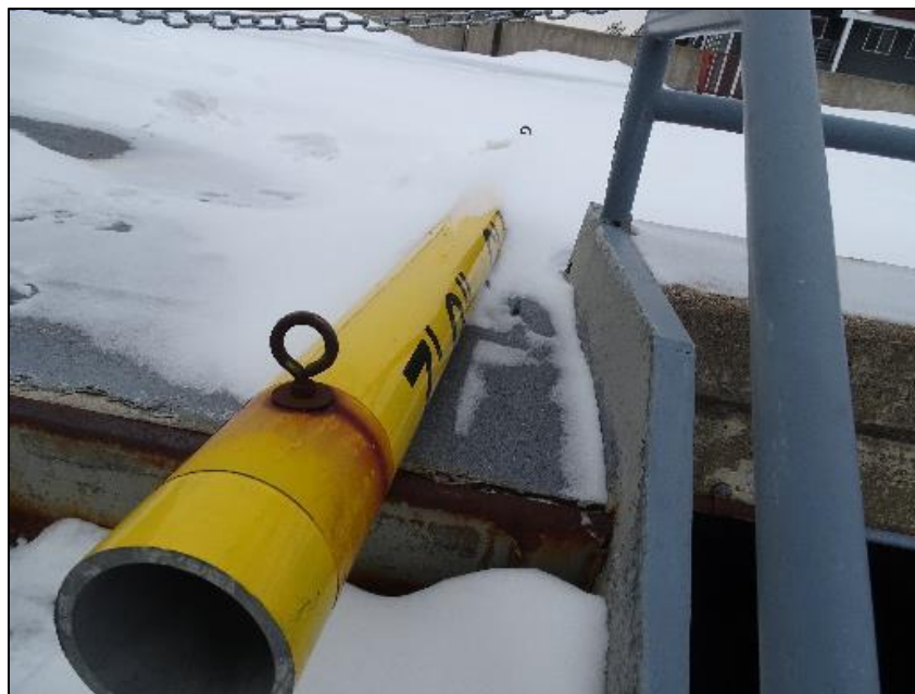
Height warning bar not installed
