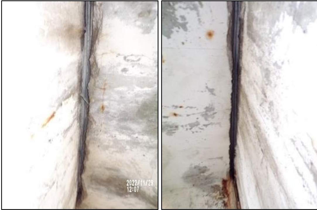
Level 3 Expansion Joint between Grid C east foundation wall on left and PT slab on right. Photo taken on Level 2
