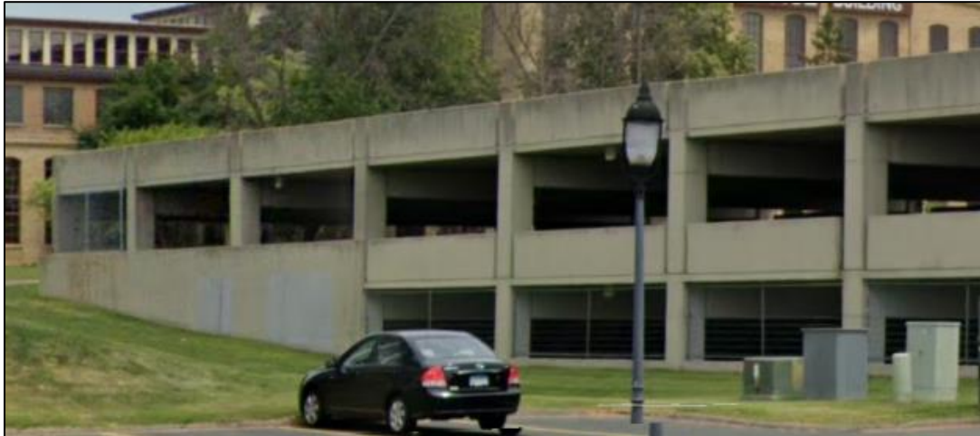
SK-7: Google Image of Northwest Corner of Levels 1 ½, 2 ½, and 3 ½. Note grade rising on north (left) end.
