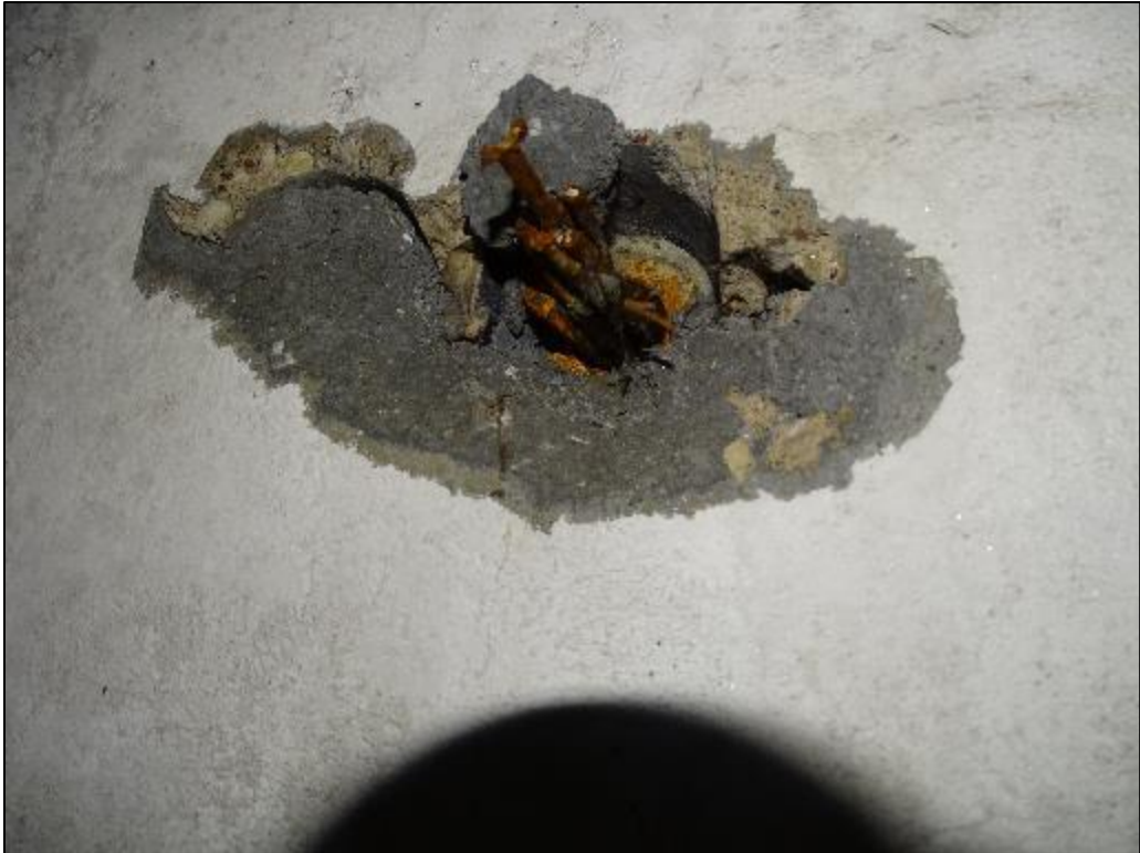
Broken PT Cable at column
