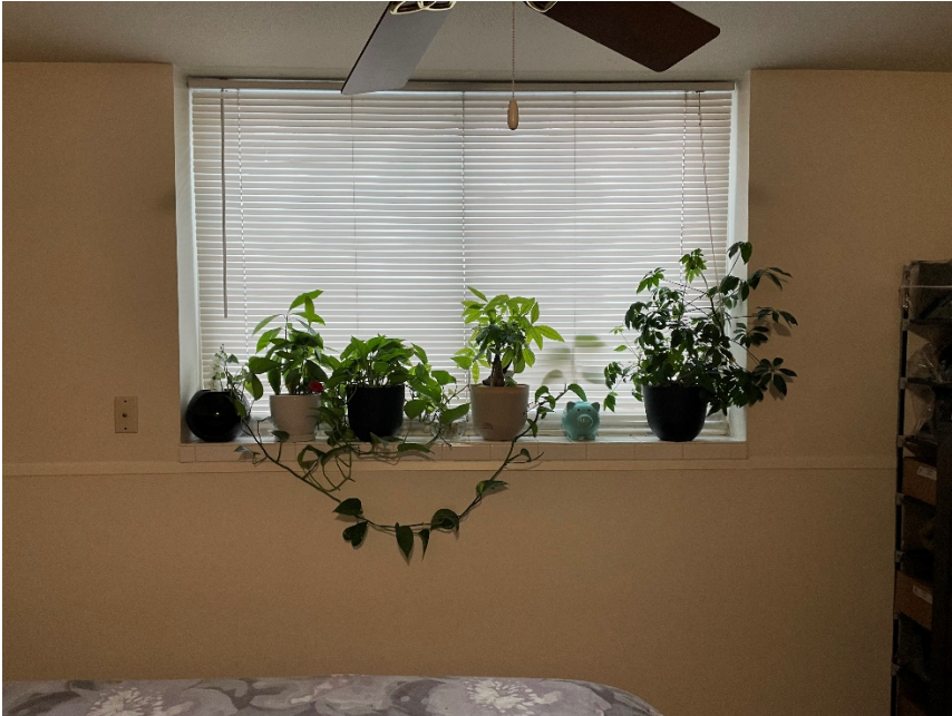
Unit 6 Window has bars on exterior but also has 2 other separate and means of escape.
