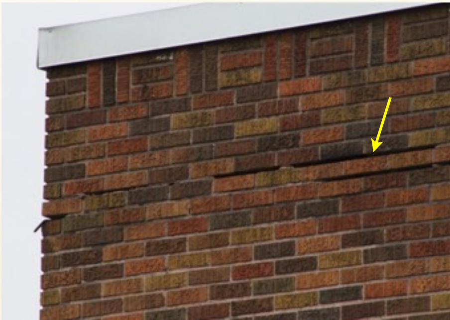
Typical joints needing tuckpointing.
