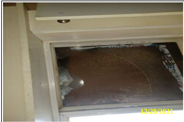
Date Serviced: 12/28/2021 Room: No Room Category: Windows
