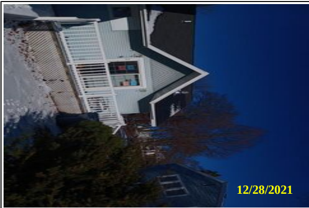
Date Serviced: 12/28/2021 Room: No Room Category: Siding
