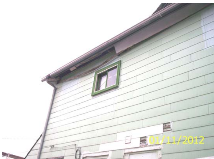
Rot damaged eave, missing siding
