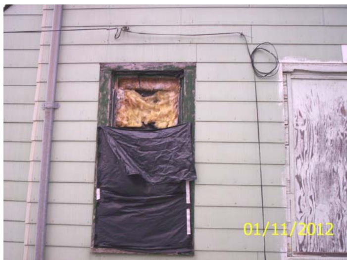
Improperly abandoned window, open wall, chipped/peeling paint
