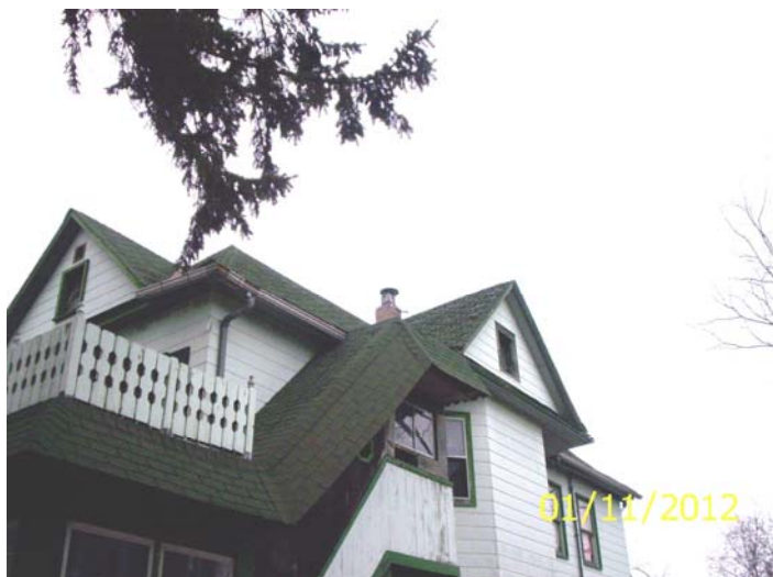
Deteriorated roof covering
