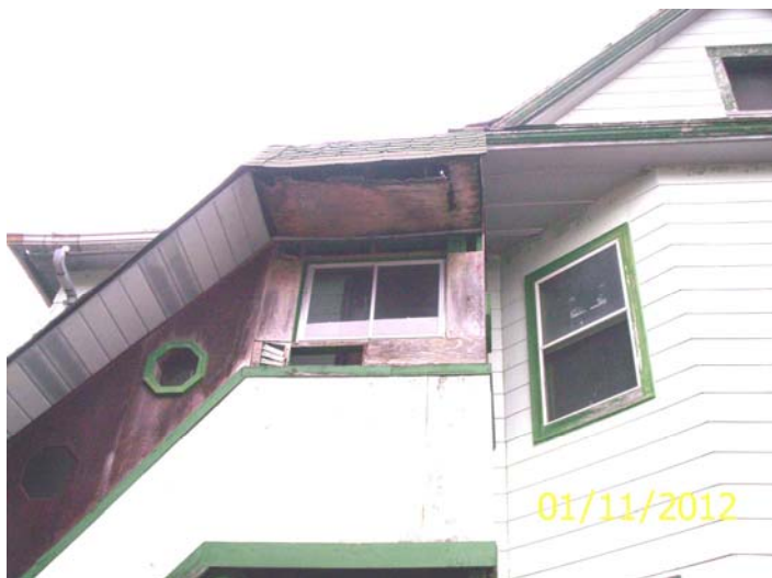
Rot damaged, open eave and wall
