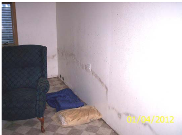
Mold in basement
