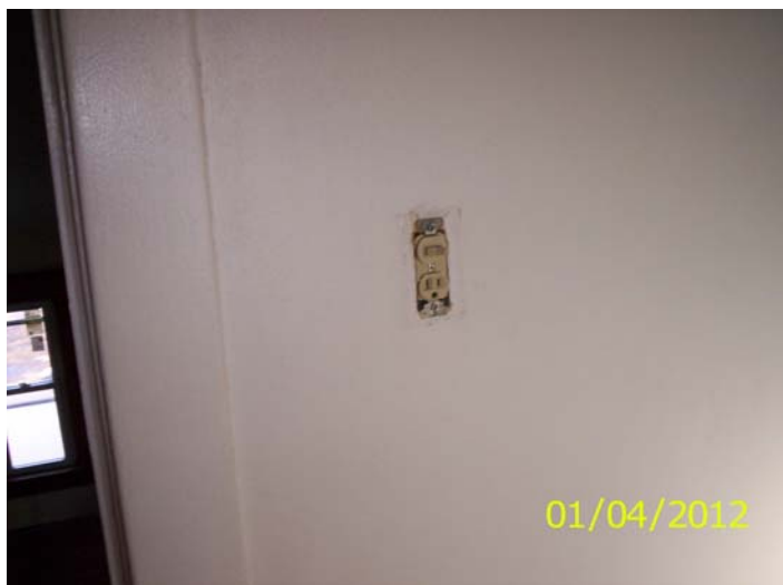
Missing cover plate; exposed wiring
