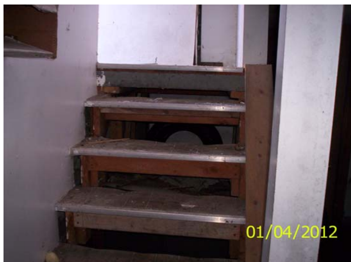
Missing hand rail for basement steps
