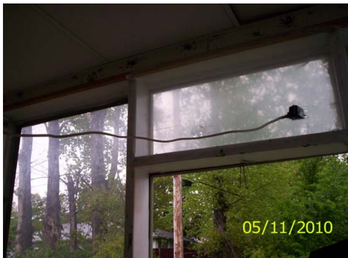
Unapproved electrical wiring on rear porch
