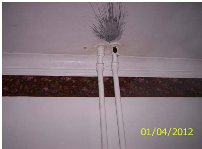
Blown out hot water heating line
