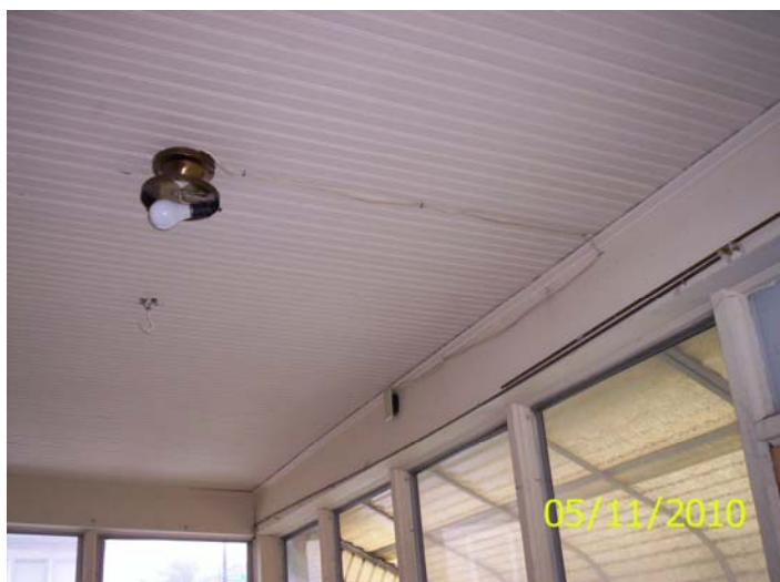
Unapproved electrical wiring on front porch
