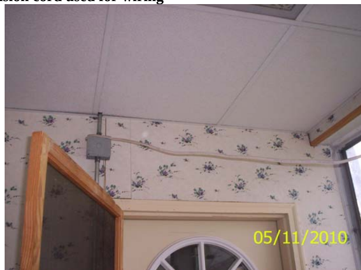
Unapproved electrical wiring on rear porch
