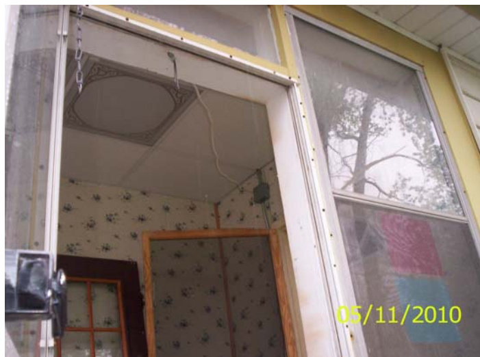
Unapproved electrical wiring on rear porch
