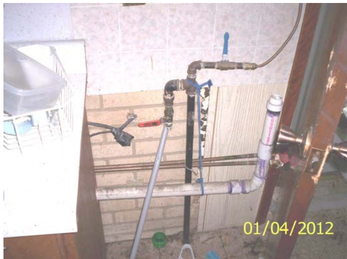
Improper electrical splice, open plumbing
