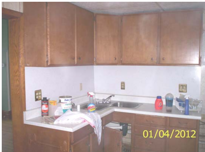
No gfc protected outlets
