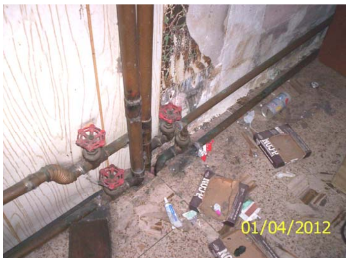
Water damaged wall, open water line, mold
