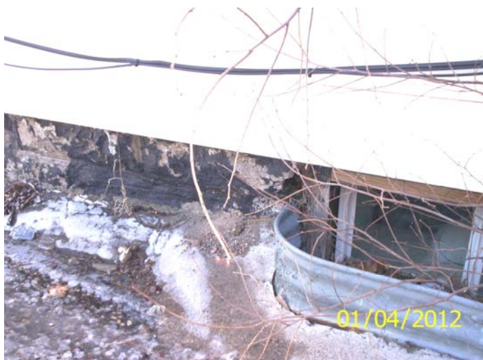
Open foundation wall, shifted block
