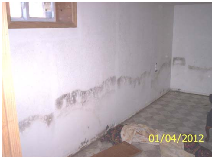
Water damaged wall, mold
