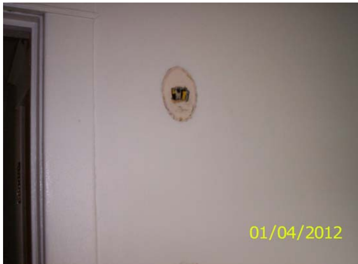
Missing fixture, open electric, exposed wiring
