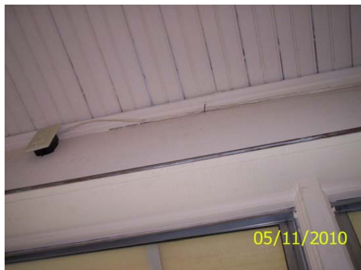
Unapproved electrical wiring on front porch
