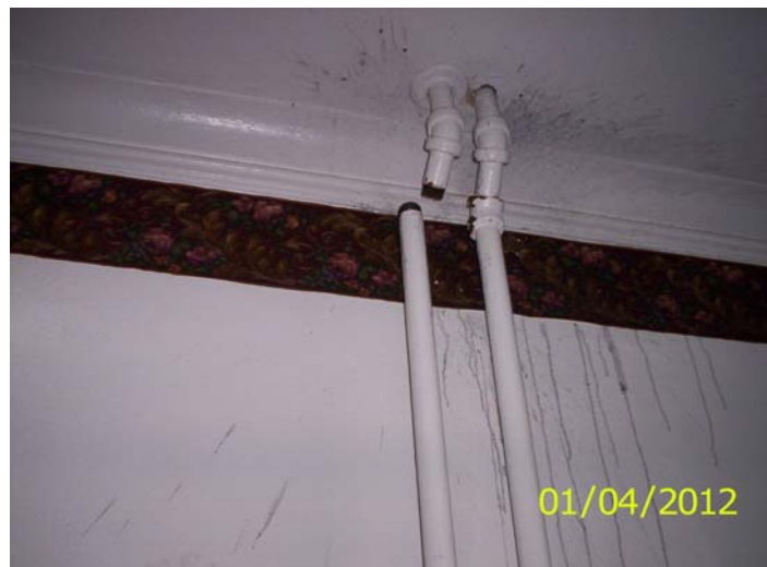
Blown out hot water heating line
