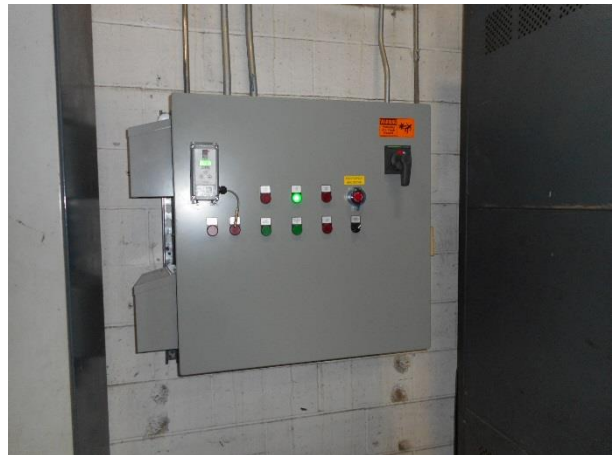
Engine Room 1 Control Panel and E-Stop
