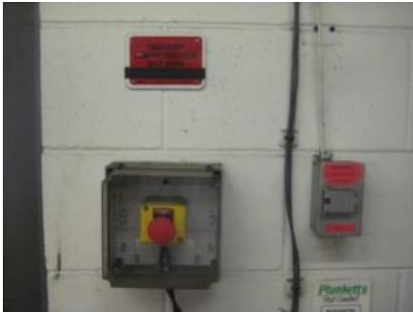
Engine Room 1 E-Stop and Manual Exhaust Control
