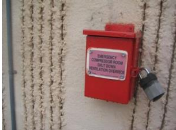
Engine Room 2 Outside E-Stop and Manual Exhaust Control
