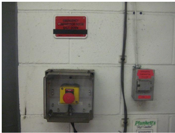
Engine Room 1 E-Stop and Manual Exhaust Control
