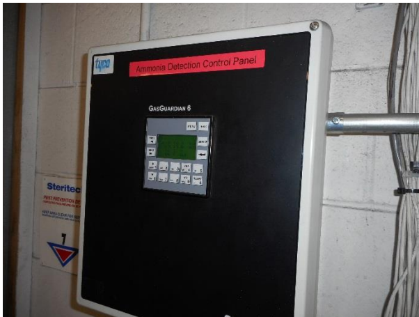
Engine Room 1 Ammonia Detection Control Panel
