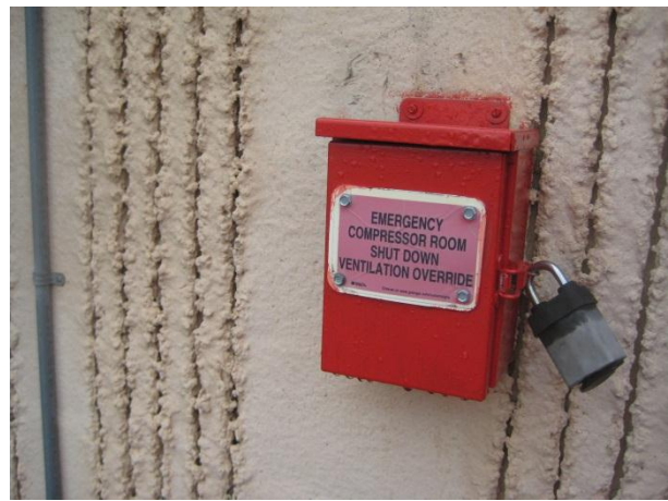
Engine Room 2 E-Stop and Manual Exhaust Control
