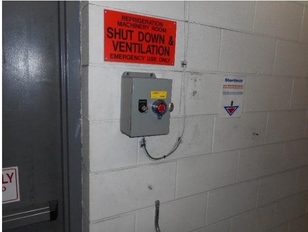
Engine Room 1 Inside E-Stop and Manual Exhaust Control
