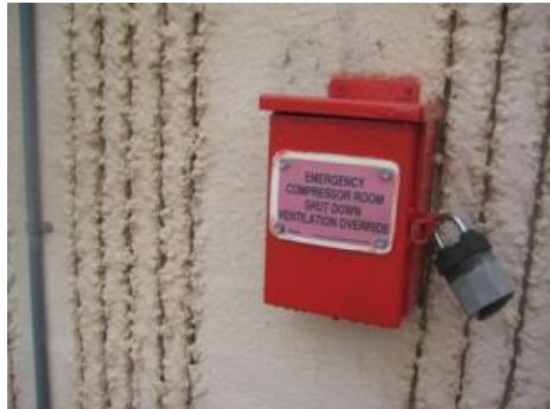
Engine Room 2 E-Stop and Manual Exhaust Control
