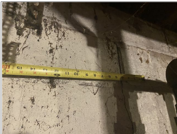
21 Minor crack in eastern basement foundation wall noted. Not a structural concern.
