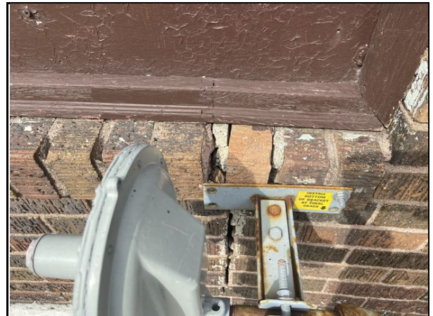
8 Cracks in brick fascia noted near gas line on east side of building. Not a structural concern.
