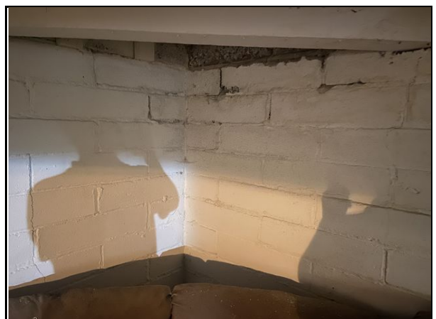
12 Minor cracking at northeast corner of basement not a structural concern.
