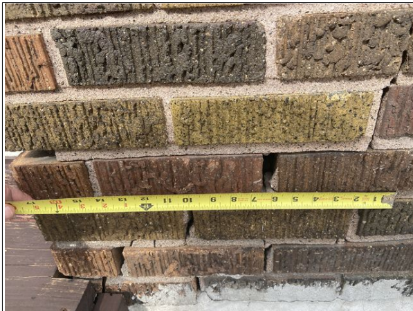
7 Cracks in brick fascia noted near gas line on east side of building. Not a structural concern.
