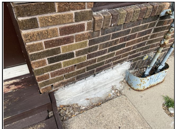
6 Cracks in brick fascia noted near gas line on east side of building.
