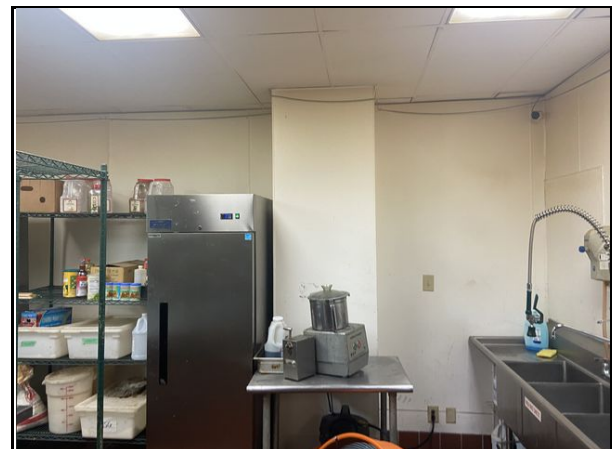
16 No structural issues noted in visible portions of eastern wall of building.
