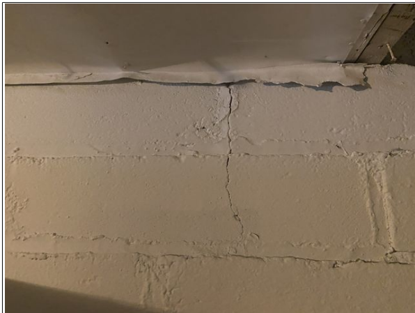
13 Minor crack in eastern basement foundation wall noted. Not a structural concern.
