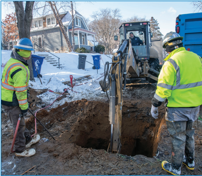
Tony Gillette, water system worker; Don Raway, HEO; and Matt Schmidt, water utility worker; replace a lead service line on Jan. 12 on Robie Street West.
