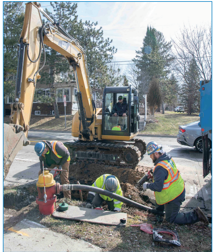
Crews work to replace a hydrant and gate at Jackson and Wheelock on April 19. From left are Aaron Erickson, Matt Schmidt, and Chris Cullen, water utility workers. The HEO is Jake Massiello. Not pictured are truck driver Jerry Lucker and supervisor Brian Gomez.
