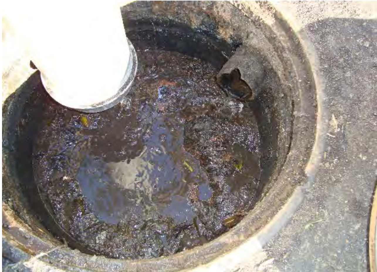
Sanitary Discharge, Private Storm Drain
