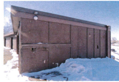
North wall deterioration
