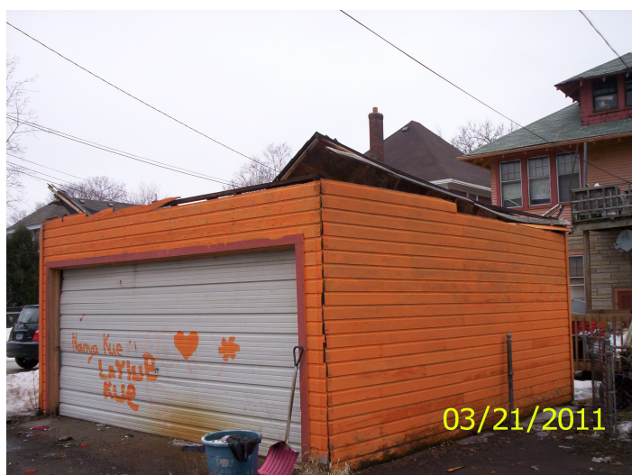
Garage, collapsed roof
