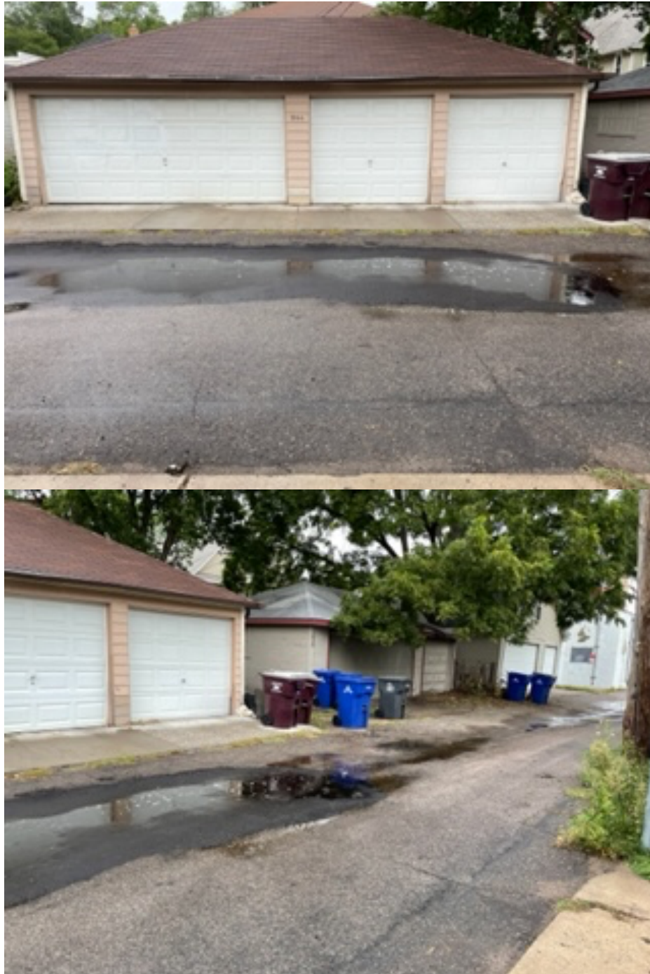
Figure 1: Alley drainage issue after minimal rainfall.
