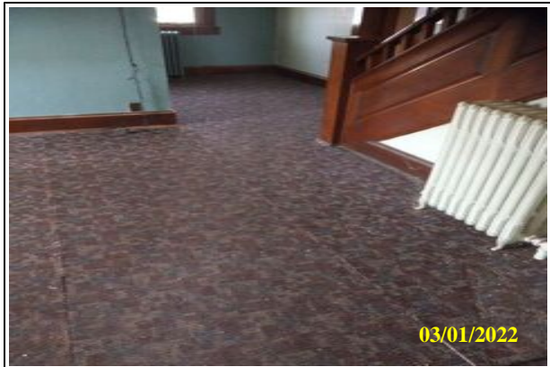
Date Serviced: 03/01/2022 Room: No Room Category: Other
